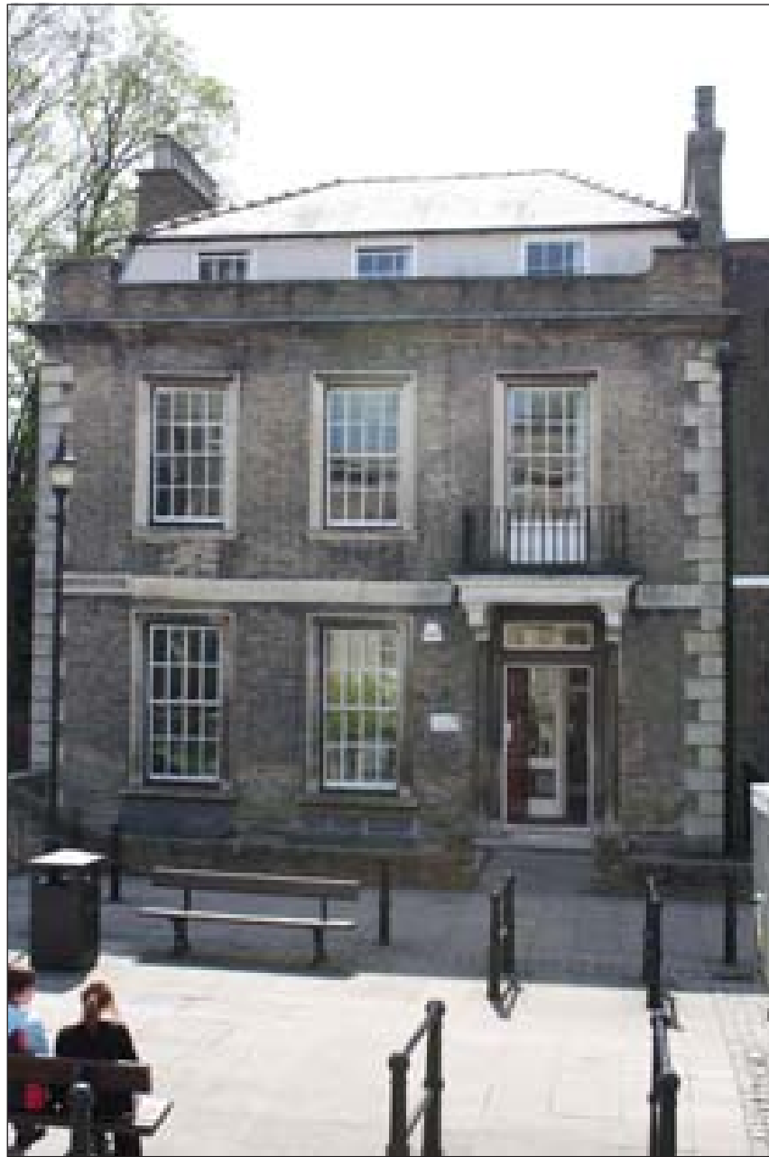
Plate 10: Building in Museum Square showing evidence of subsidence, possibly into moat below
